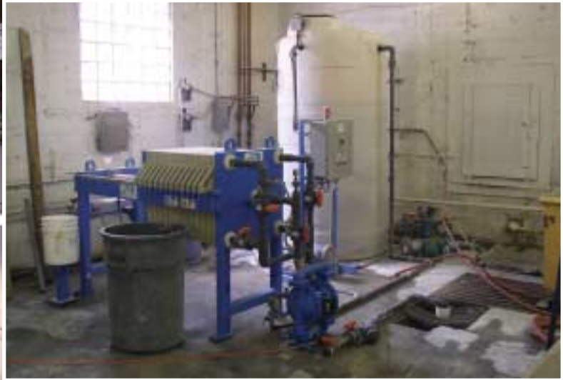
Water is recycled in the facility with a water treatment system manufactured by Water Treatment Technologies.
