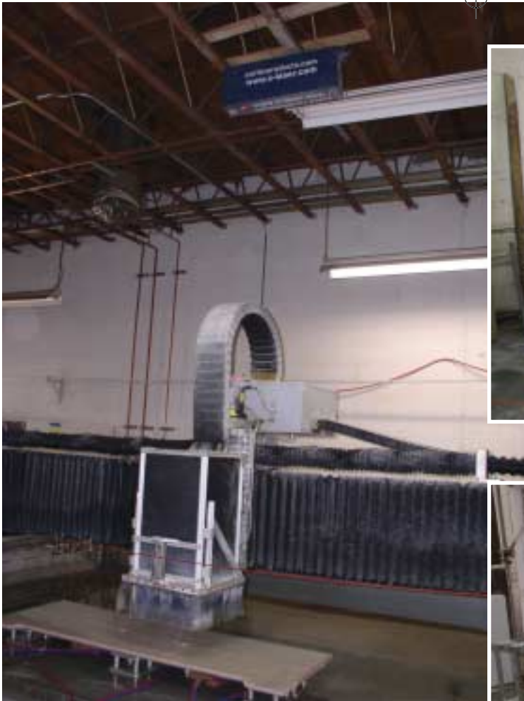
Three months after the CNC machine was installed, a Z-laser positioning system from Carter Products was installed above it to minimize errors in fabrication.
