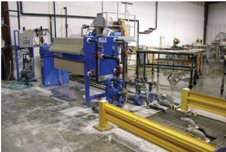
One of the most recent additions to Down East Fabrication's stone shop is a water treatment facility from Water Treatment Technologies in Hampton, NH.
